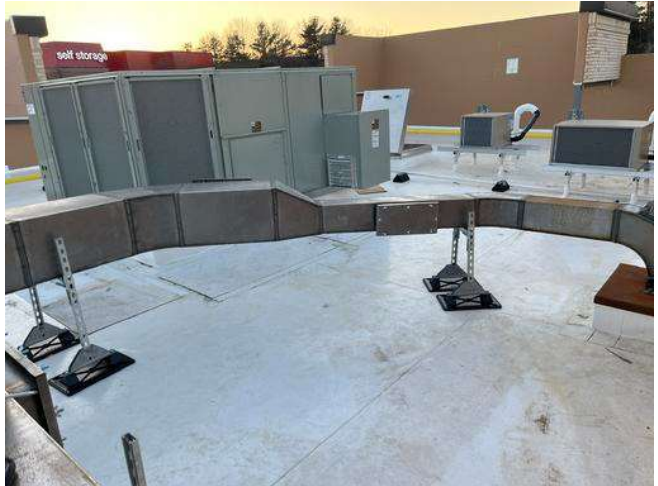
Grease Duct Supports
